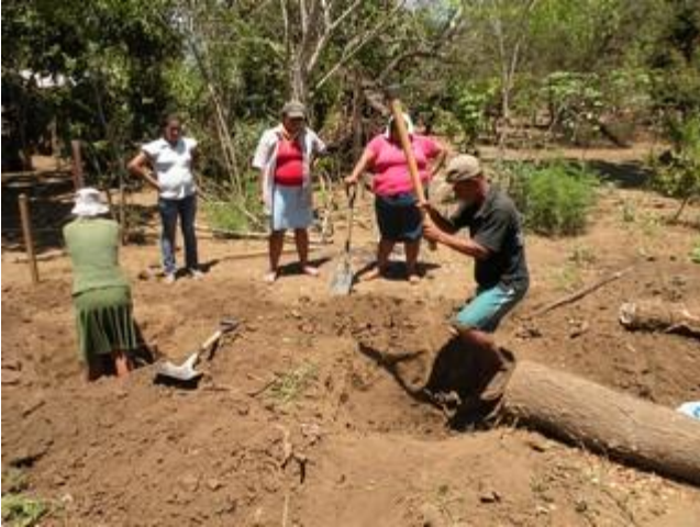
The community in Monte Olivo working hard at removing stumps on the site of the future Shirley Case School.
